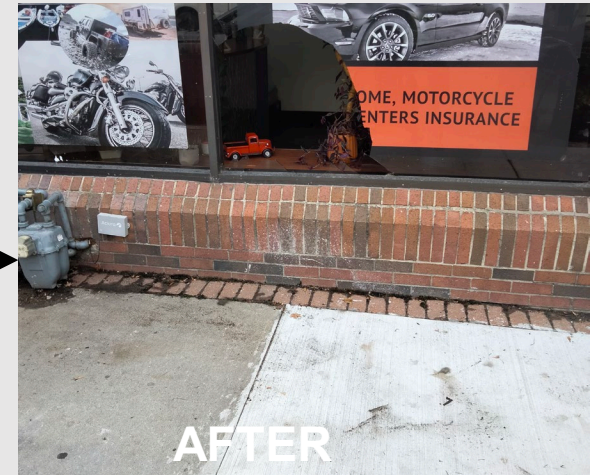
Broken Glass Picked Up
